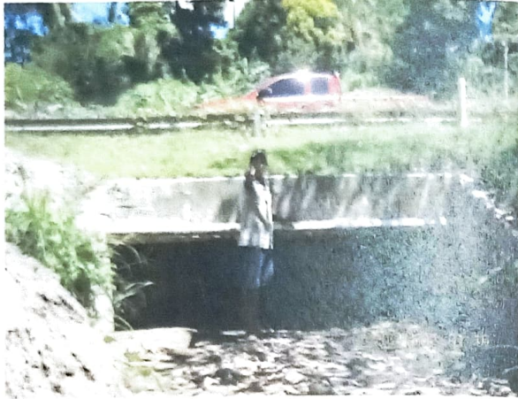
Figure 9.2: A sub-surface drain mainly with re-enforcements such as plastic or concrete material
